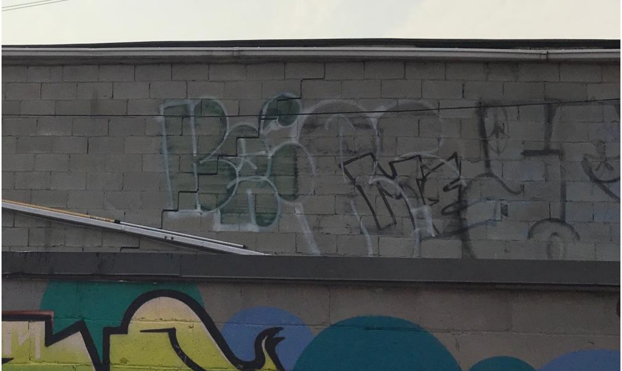
Figure 8 Close up view of east wall showing saw tooth crack in wall
