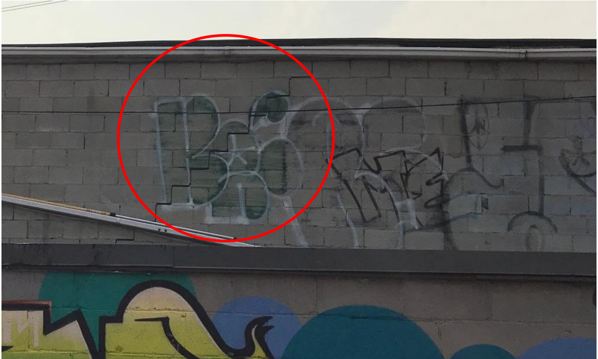
Figure 3 Close up view of east wall showing saw tooth crack in wall
