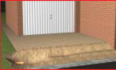
1. Excavate to allow room for channels/catch basin and 4" of concrete on all 3 sides.
